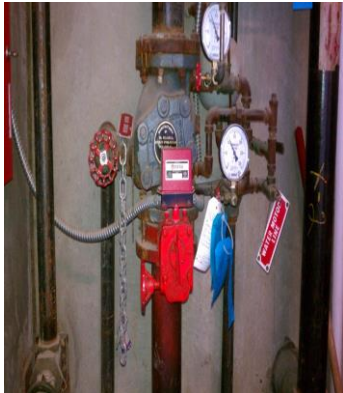
Riser Room Sprinkle System
