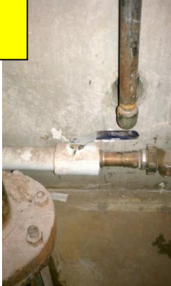
Riser Room Water Shutoff
